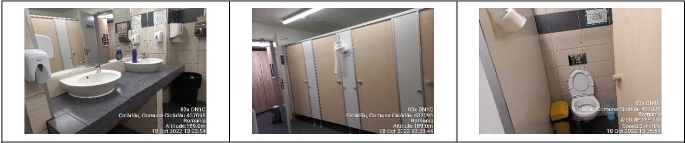
Washing hands and toilet area
